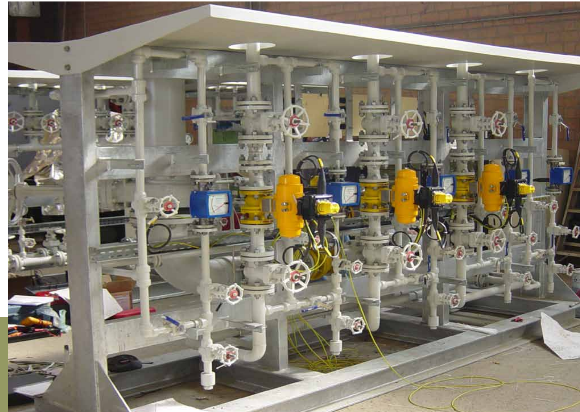
Pilot Gas / Purge Gas Skid Petrochemical plant, UAE
