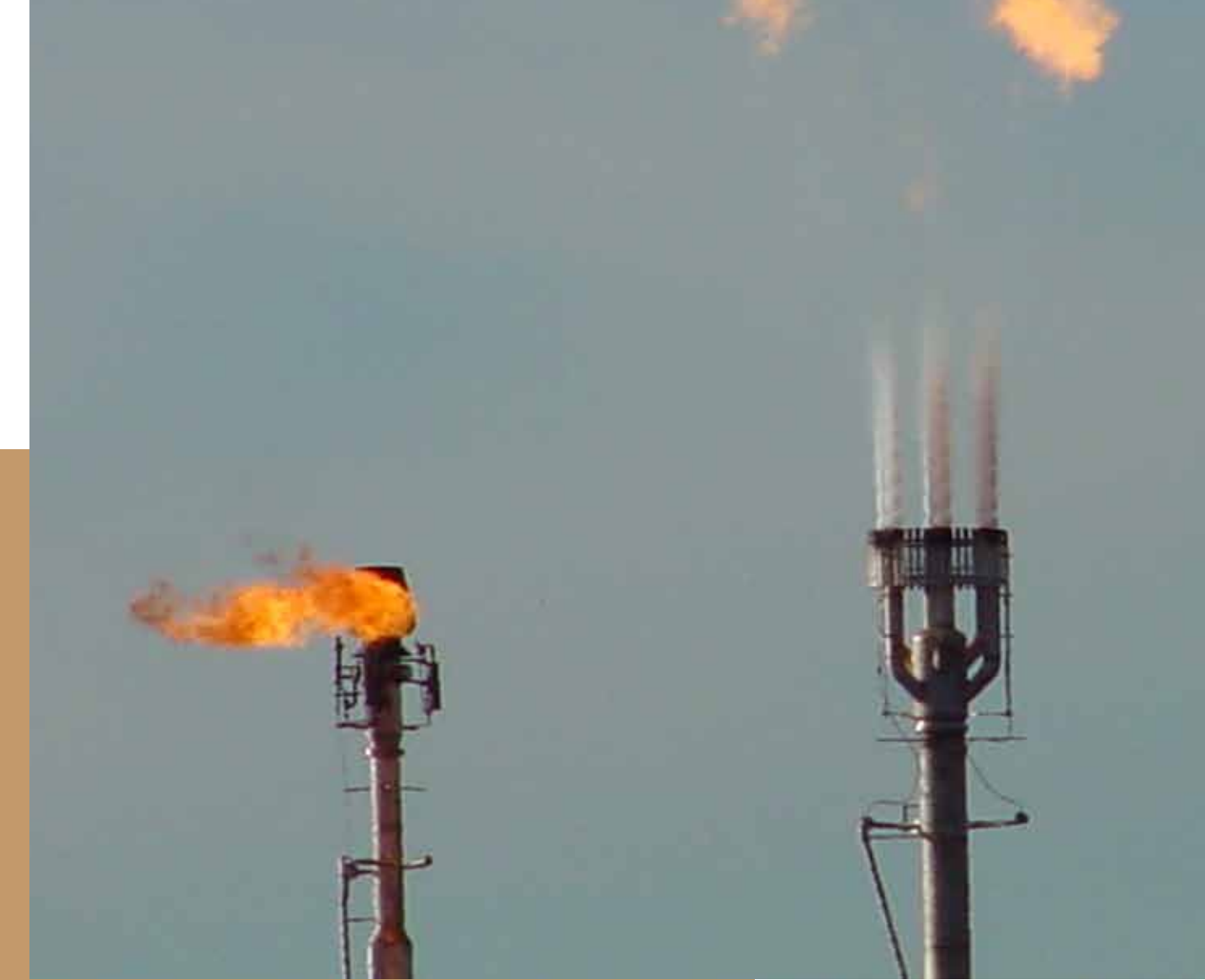
CSF-7-14 Flare Tip Gas plant Alaska
