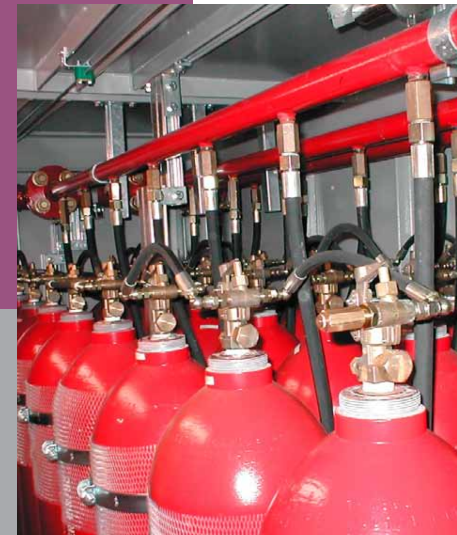
CO2 Snuffing System Offshore Nigeria
