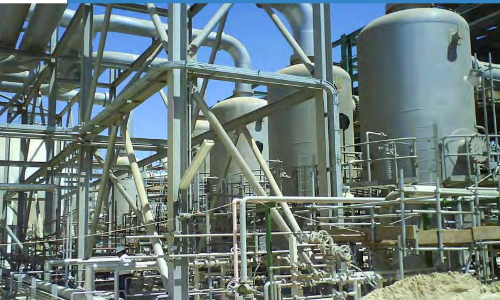
Water Seal Drums Petrochemical plant, Saudi Arabia
