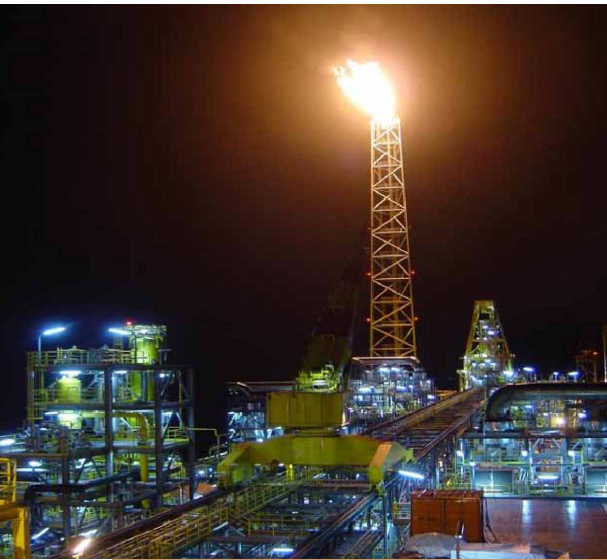
CSF-6-8-HL-14 HP/LP Flare Tip FPSO offshore Nigeria
