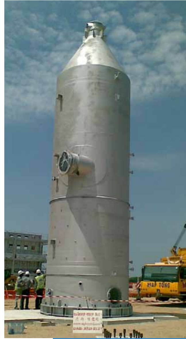
Vertical Knock-out Drum Refinery, Singapore
