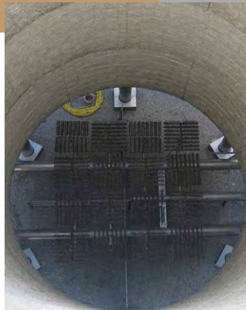
Looking down onto GFIN EGF Ground Flare Burner Matrix Mugardos, Spain
