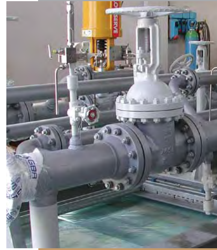
Steam Control Skid Petrochemical plant UAE
