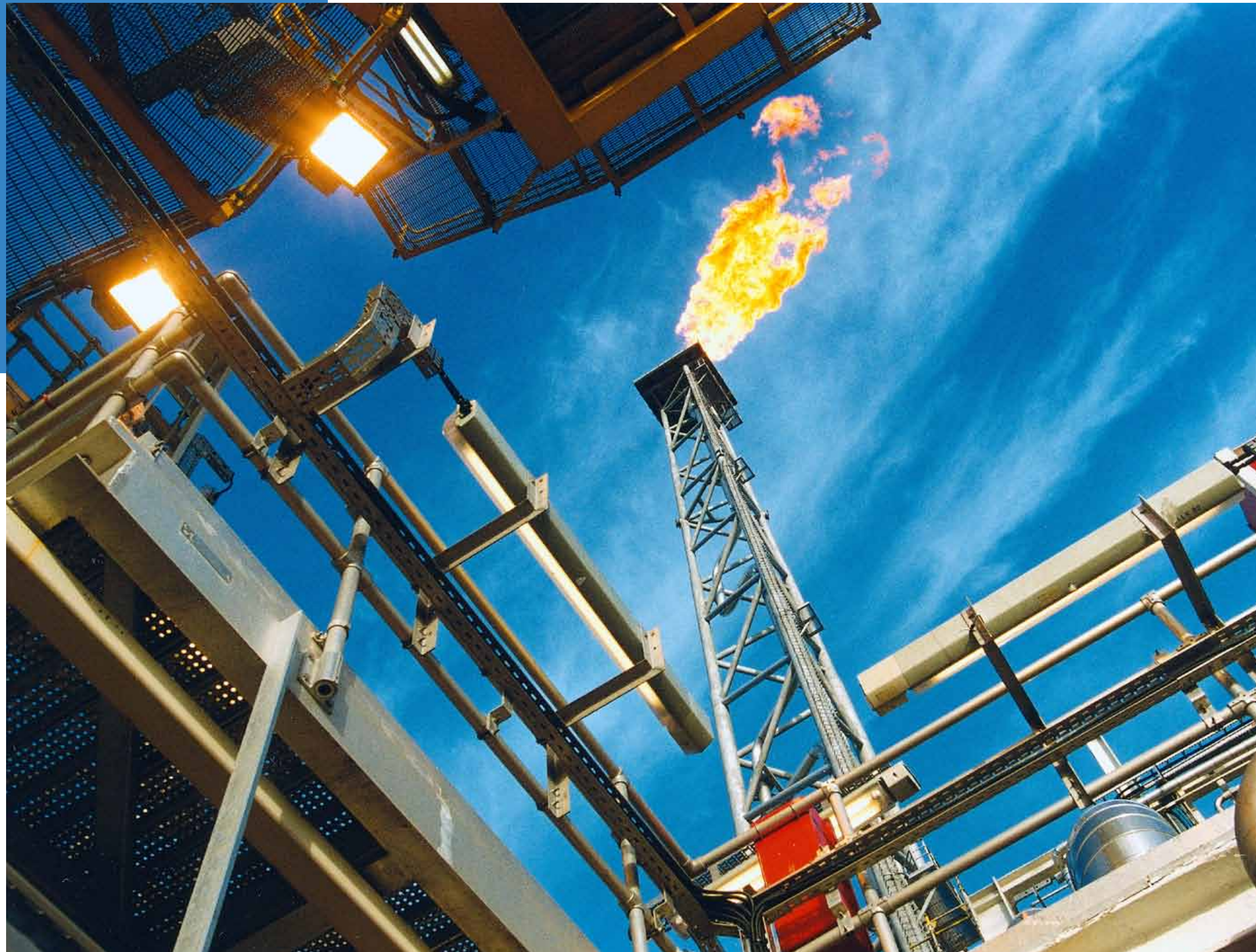
CSF Flare Tip in operation on an FPSO
