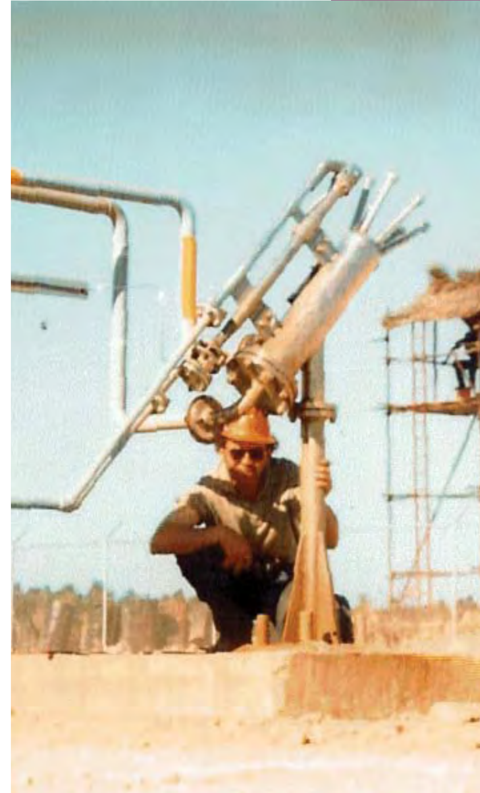
Smokeless Liquid Condensate Burner Onshore oil and gas terminal
