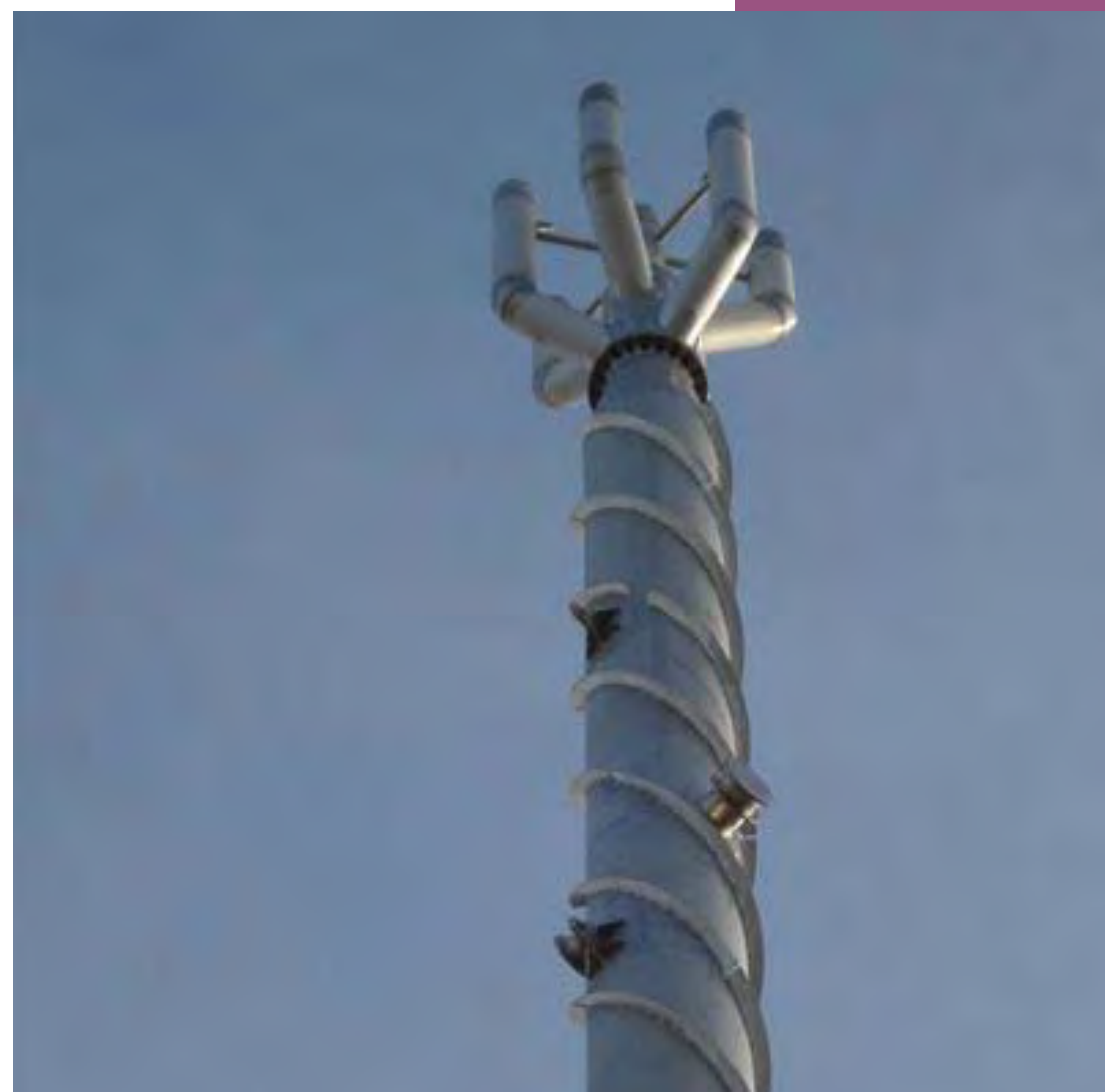
CSV-7-10 Vent Tip Underground gas storage project, Germany
